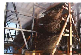
“Yumetake (bamboo cooling system) at Hyotan Onsen”
